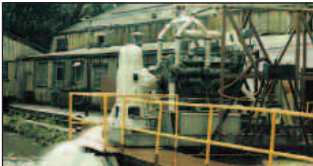
RB 2.15 flywheel mounted coupling on a Detroit Diesel driven Peerless pump
