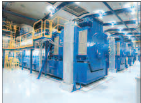
Natural gas powered wartsila generator sets.
